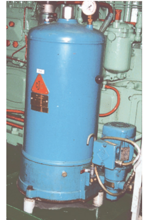
HDU2 27/54 P for lube oil treatment
