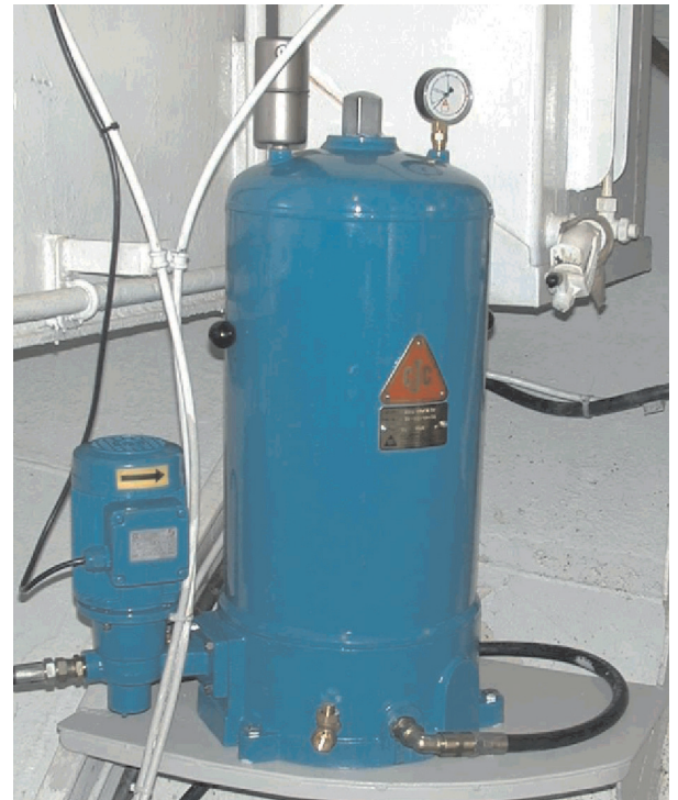
The CJC™ Fine Filter installed in the engine room
